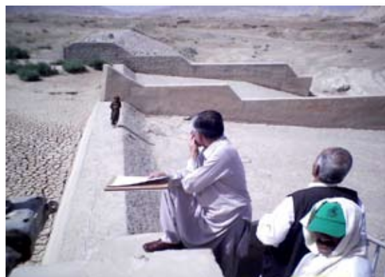
Figure 2 Weir structure, head regulator and canal at Shabo Headworks, Pishin district, Balochistan.
